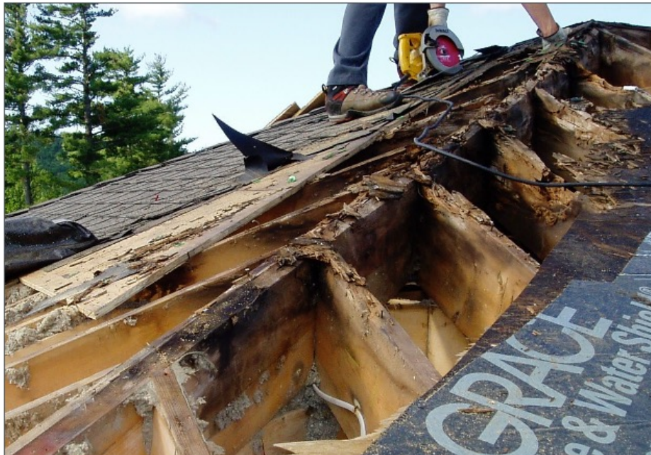
Image 03 - Wood rot in a roof caused by air exfiltrating from the inside of the building to the outside. The moisture carried by the air caused permanent damage to the roof structure.
